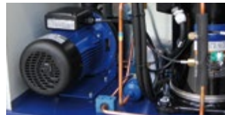
Pump P3 (3 barg) / P5 pump (5 barg, optional).
